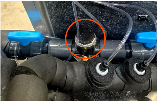
Typical Spa Set Up
